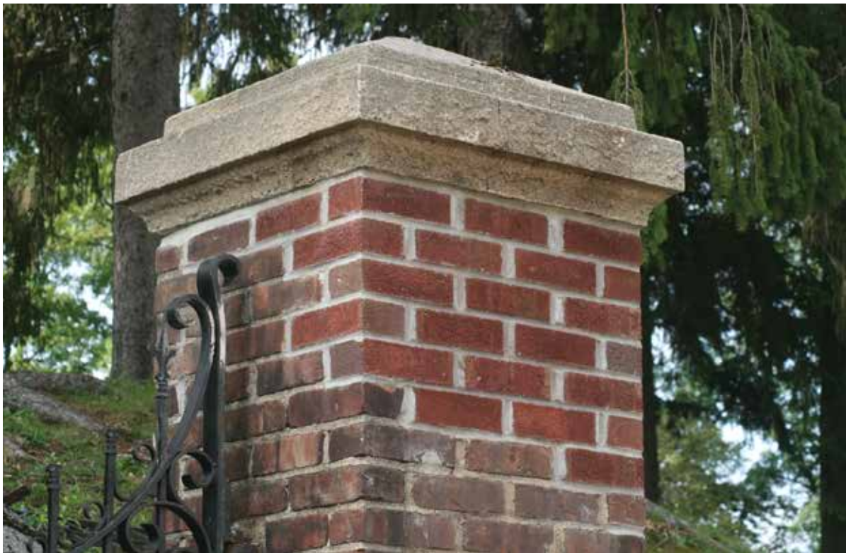
These three photos of the three restored brick columns, taken on September 25, 2011, provide a comparison of the old and the new bricks and mortar. The new bricks are the same dimensions as the old bricks, and they duplicate the alignment of the old bricks. The juxtaposition draws attention to deterioration of the 82-year-old masonry. The flat slate capstones on the outer columns do not match the original cement pyramidal capstones that they replaced.
