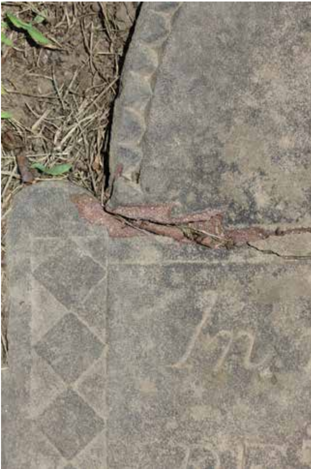
1808: Peter Bilyeu cut by Henry Sillcocks A crack reveals the natural red color of the sandstone.
