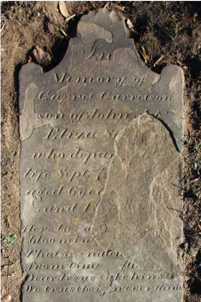
1820: Garret Garretson Sebring unknown stonecutter. Part of the top layers are gone from this otherwise legible stone. No impression of carving remains in the delaminated section.
